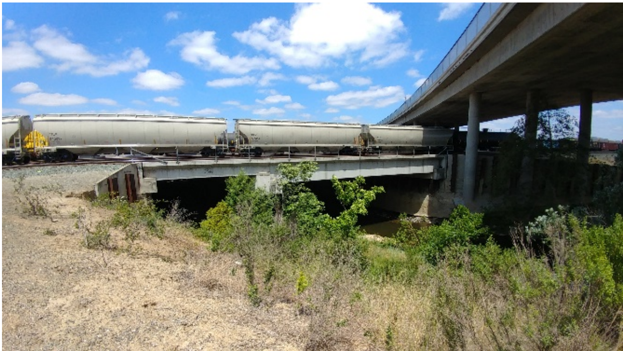
Photo 2-7: Foothills Blvd. and UP Railroad Yard bridges over Dry Creek, looking north.
